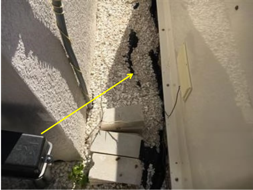
Photo 48- erosion at equipment area
