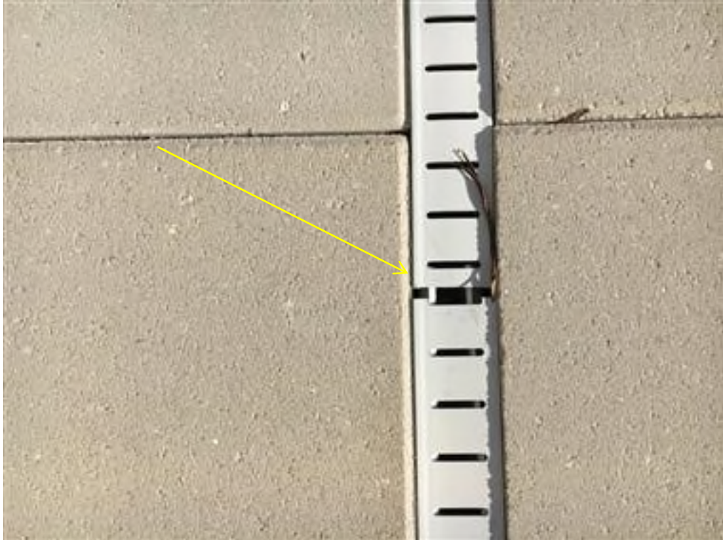
Photo 9- pool deco drain
