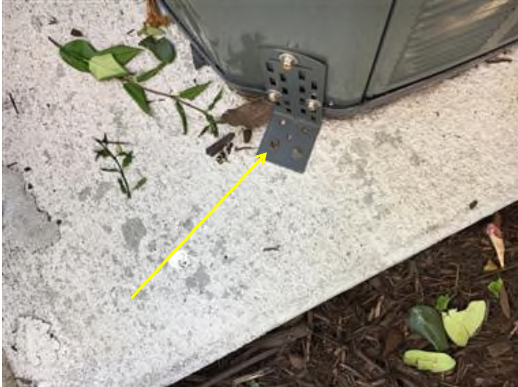
Photo 51- AC tie down
