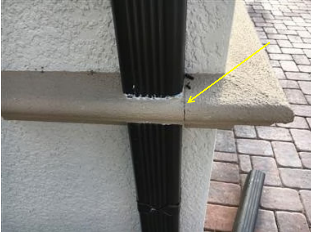
Photo 101- open trim joint 9836 Haze Drive
