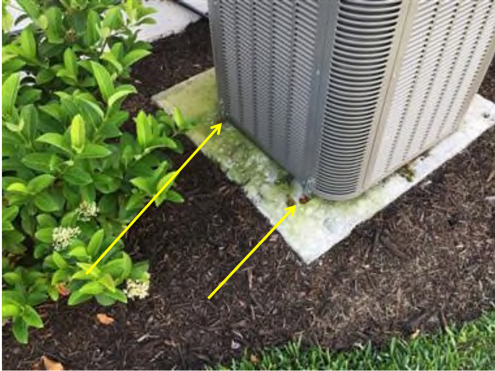
Photo 104- AC tie downs typical, 9835 Haze Drive
