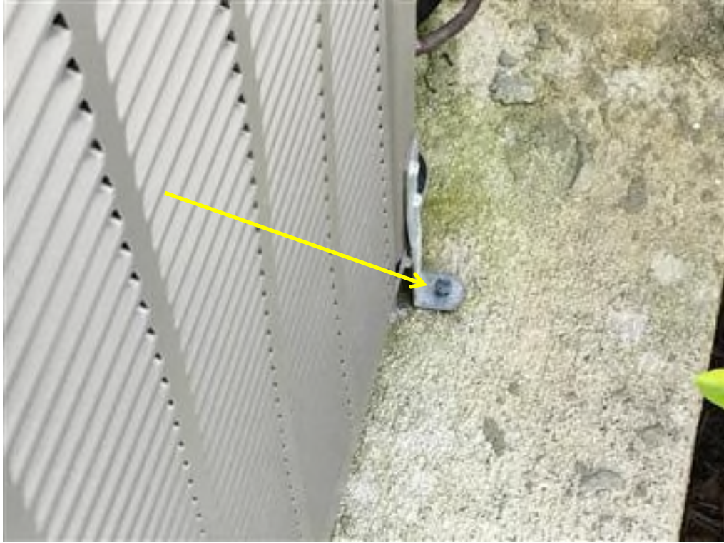
Photo 106- AC tie downs typical 9835 Haze Drive
