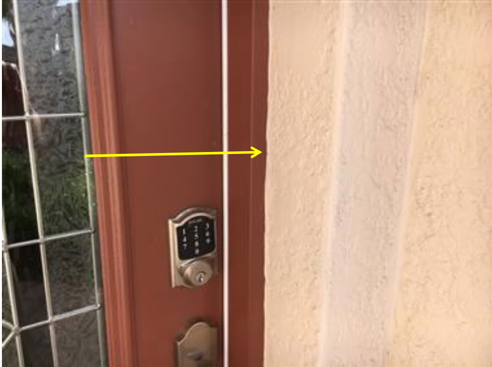
Photo 103- sealant at door typical, 9835 Haze Drive
